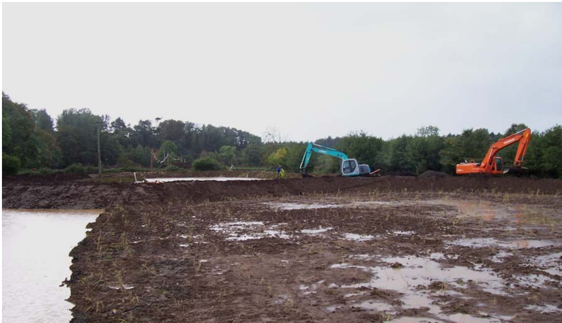
Figure 7 Phragmites australis (Common reed) planted in Pond 1. The excavators in the background were completing bank formation and levelling topsoil
